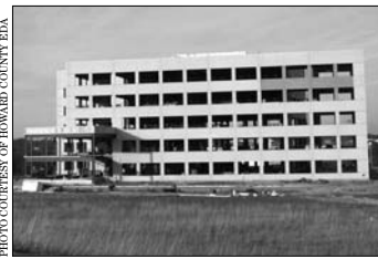
Under construction: Merkle’s new 120,000 square-foot, build-to-suit Class-A office building in the Columbia Gateway Business Park.
